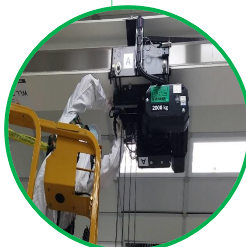
Cleanroom Overhead Crane Maintenance
