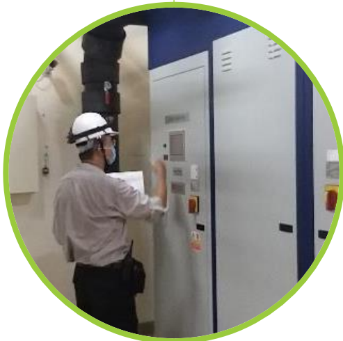
Operation of N2 Gas Purification Equipment
